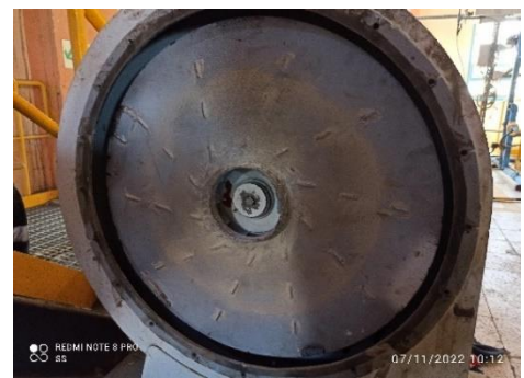
Figure 11. Fan after cleaning
